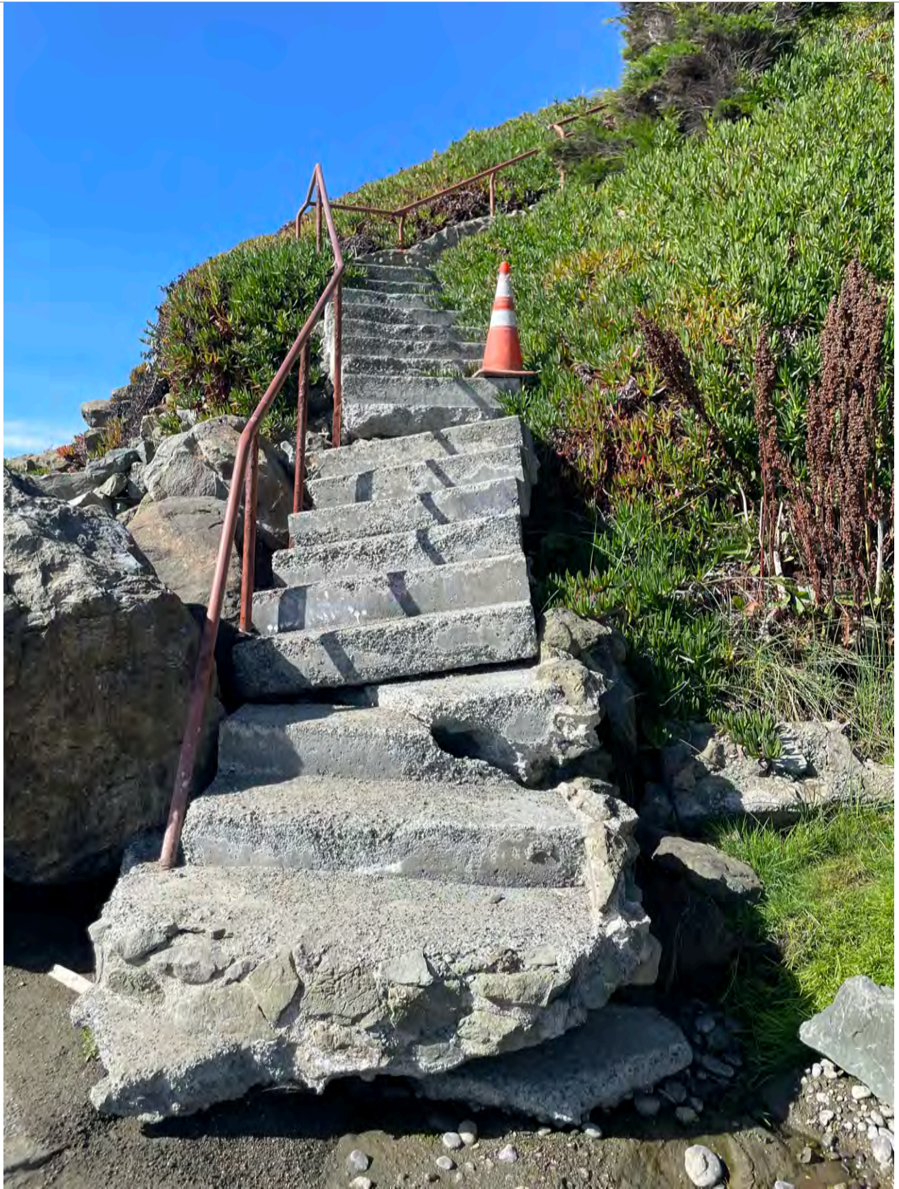
Photo 2. View from the base of the Surfer Stairs showing severe damage to the lower 11 steps at the mudstone outcropping, photographed September 23, 2026.
