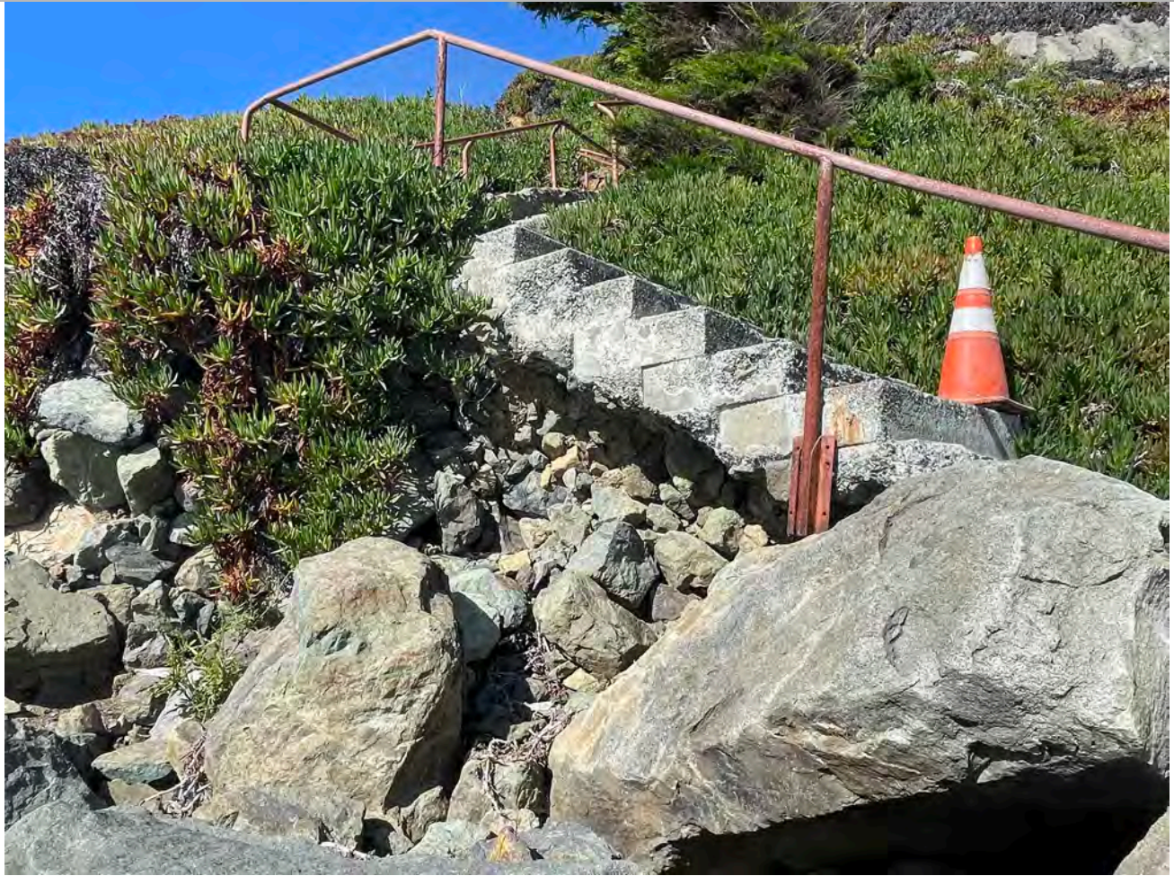
Photo 3. View of the lower stairs showing loss of supporting material beneath at least six stair treads and displacement of adjacent rock material.
